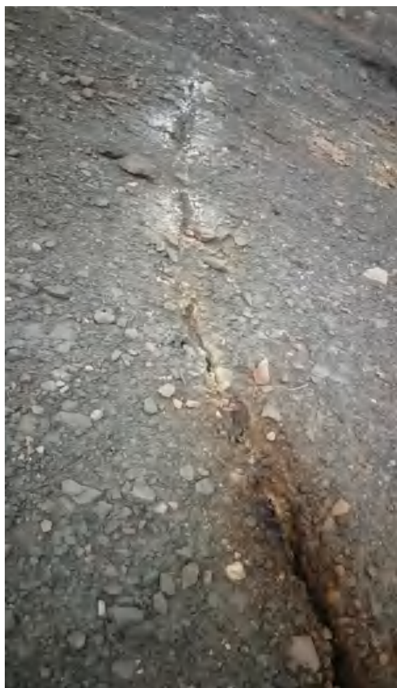
Figure 20: Fume cracks in the Bhulanbarari area.
